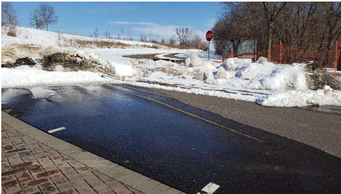
Figure 46. Permeable Pavers: Intercept Meltwater Where Asphalt Conveys It
