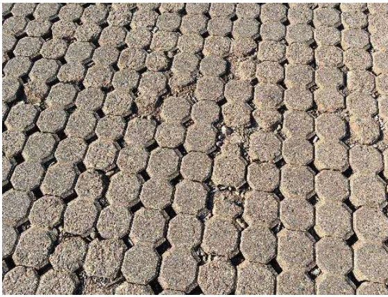
Figure 47. Salt Erodes Many Surfaces, Including Pavers
