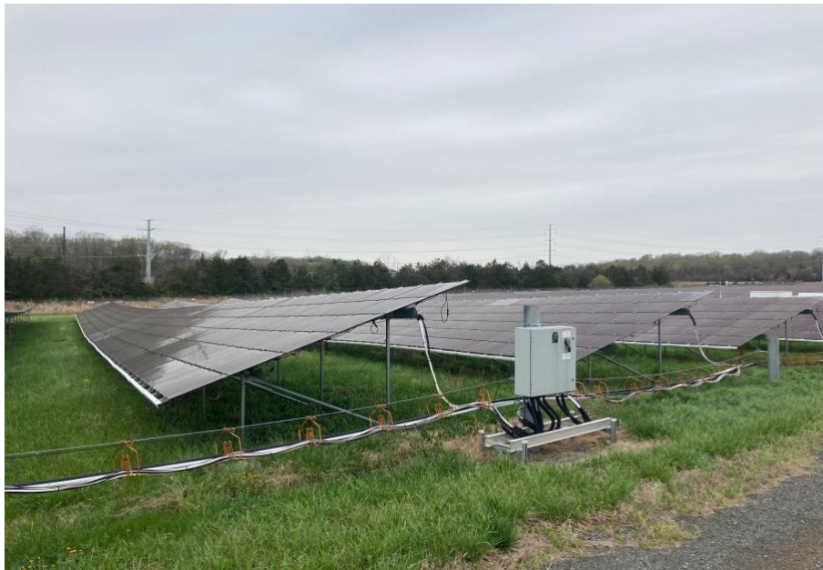
Figure 9. Participants visited a solar site in Remington and were provided a tour of the project by Sterling Turner (Dominion Energy).
