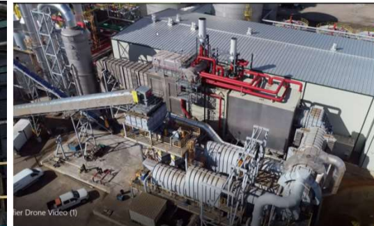
15,000 TPY + 7 MWe+steam ICMInc.com
