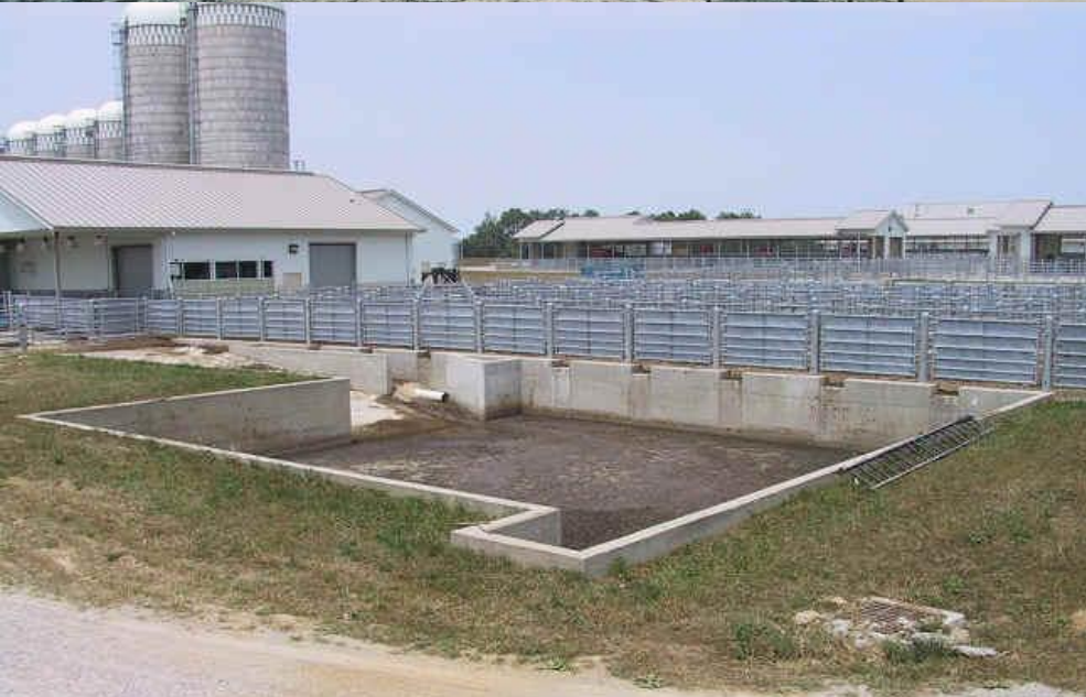
Gravity Settling Basin
