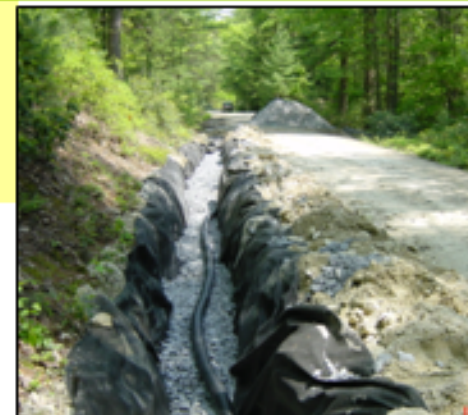
This underdrain collects water from springs and seeps under the road ditch.
