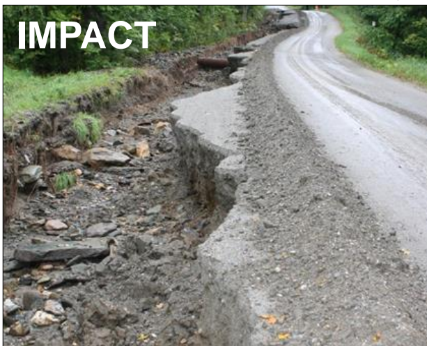
Eroding roadside ditch
